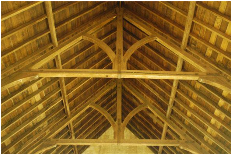
Above: the Balmain roof; below: the Berrima roof (Images: Brian Andrews & Ian Stapleton)
