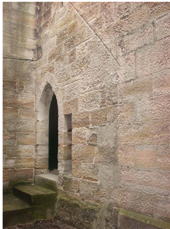
Site of the demolished sacristy (Image: Jude Andrews)
